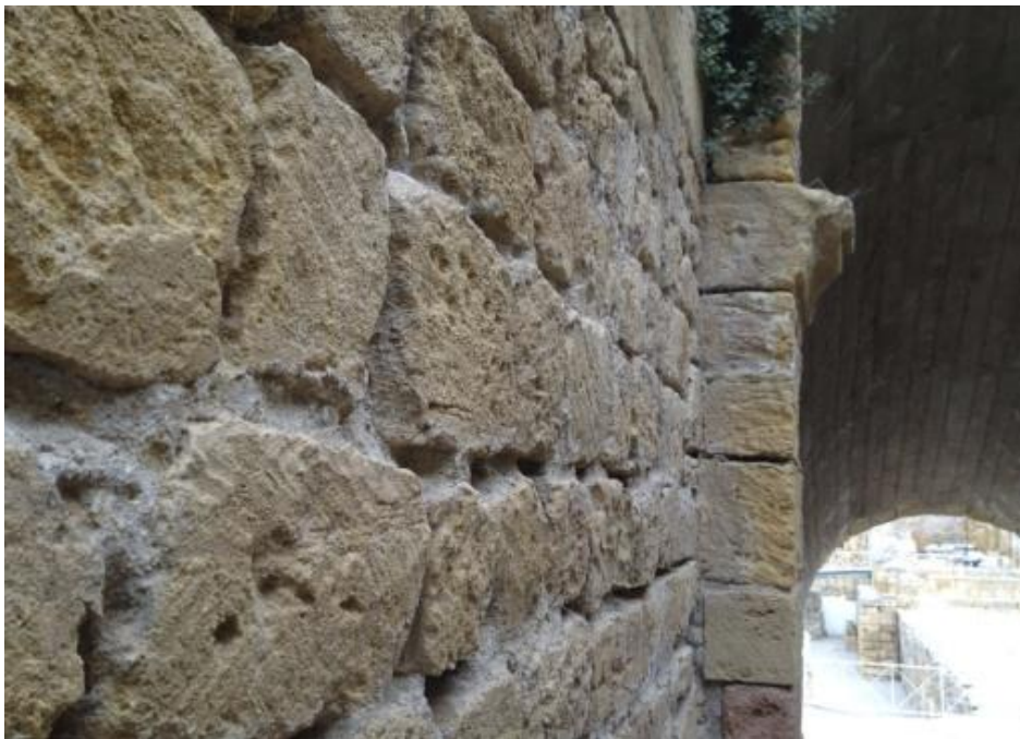
Figure 9. Efflorescing, The Archaeological Ensemble of Tárraco (Spain)
